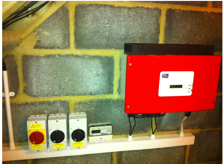
Above: showing AC/DC isolators, energy meter and inverter housed inside the garage
