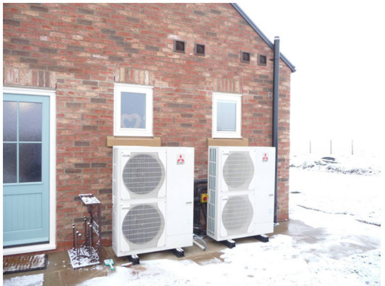
Above: showing two 14kW Mitsubishi Ecodan Air Source Heat Pumps
